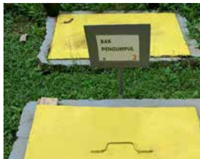
Bak Pengumpul 2 : Sumber limbah dari gedung utama dan sumber limbah dari bekas air wudhu mushola Collecting Tub 2: Waste source from the main building and the source of waste from the ex-water ablution prayer room
