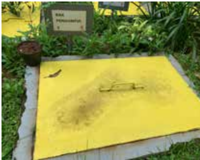
Bak Penumpul 3 (4) : Sumber limbah dari gedung utama dan sumber limbah dari bekas air wudu mushola dan dari septictank biofilter mushola Bathtub Collector 3 (4): The source of waste from the main building and the source of waste from the former wudu water mosque and from septic tank biofilter mushola
