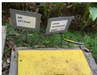
Air Lift Pump & Aerob Sedimentasi akhir 11: proses sistem biofilter aerob 3 dan proses sedimentasi akhir dan resirkulasi air lift pump. Air Lift Pump & Aerob Sedimentation end 11: process of aerobic 3 biofilter system and final sedimentation process and recirculation of water lift pump.
