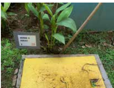
Aerob & Aerasi 10 : Proses sistem biofilter aerob 2 dan proses aerasi 2 Aerob & Aeration 10: Process of aerobic 2 biofilter systems and aeration processes 2
